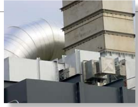
Secondary heat recovery system returns energy to process or other plant energy requirements
